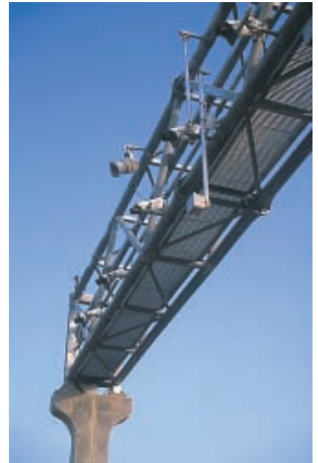
Tolling gantry showing the all-electronic tolling technology used on the Cross Israel Highway
