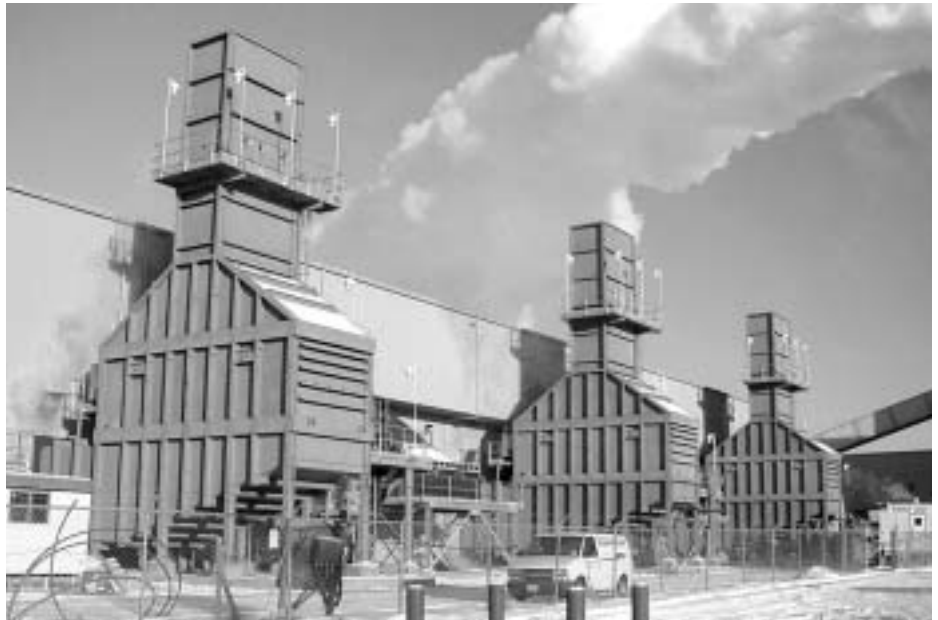
Three of the six OTSGs installed at the Queen Elizabeth Power Plant in Saskatoon, Saskatchewan. The units provide steam for an energy efficient and environmentally friendly cogeneration plant.
