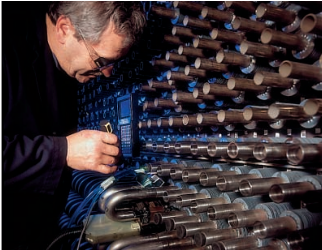
Pressure parts being installed during the final assembly of an OTSG module. Each tube connection is welded using IST's highly specialized orbital welding system.
